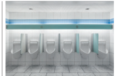
↑ Before: These old urinals have become prone to faults and are causing a lot of maintenance work.
