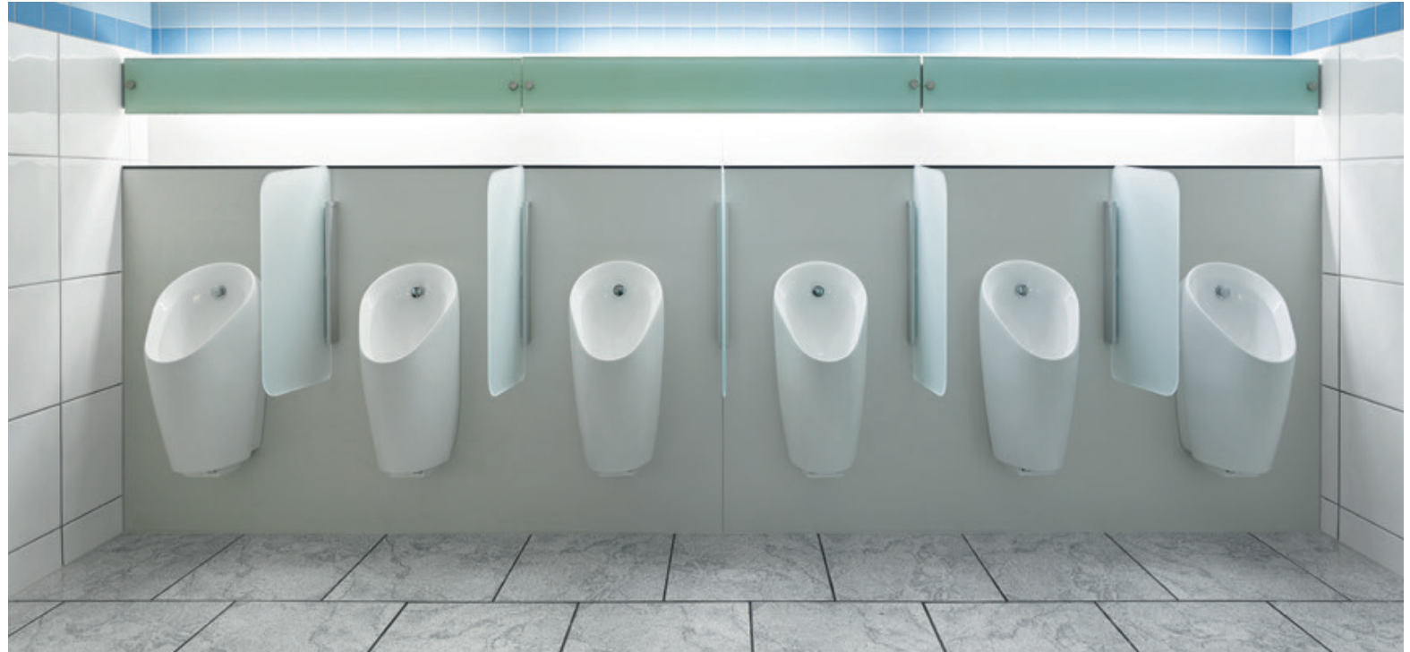
↑ After: The partial renovation of this toilet facility sees six new Geberit Preda urinals and Geberit urinal divisions installed in just four days.
