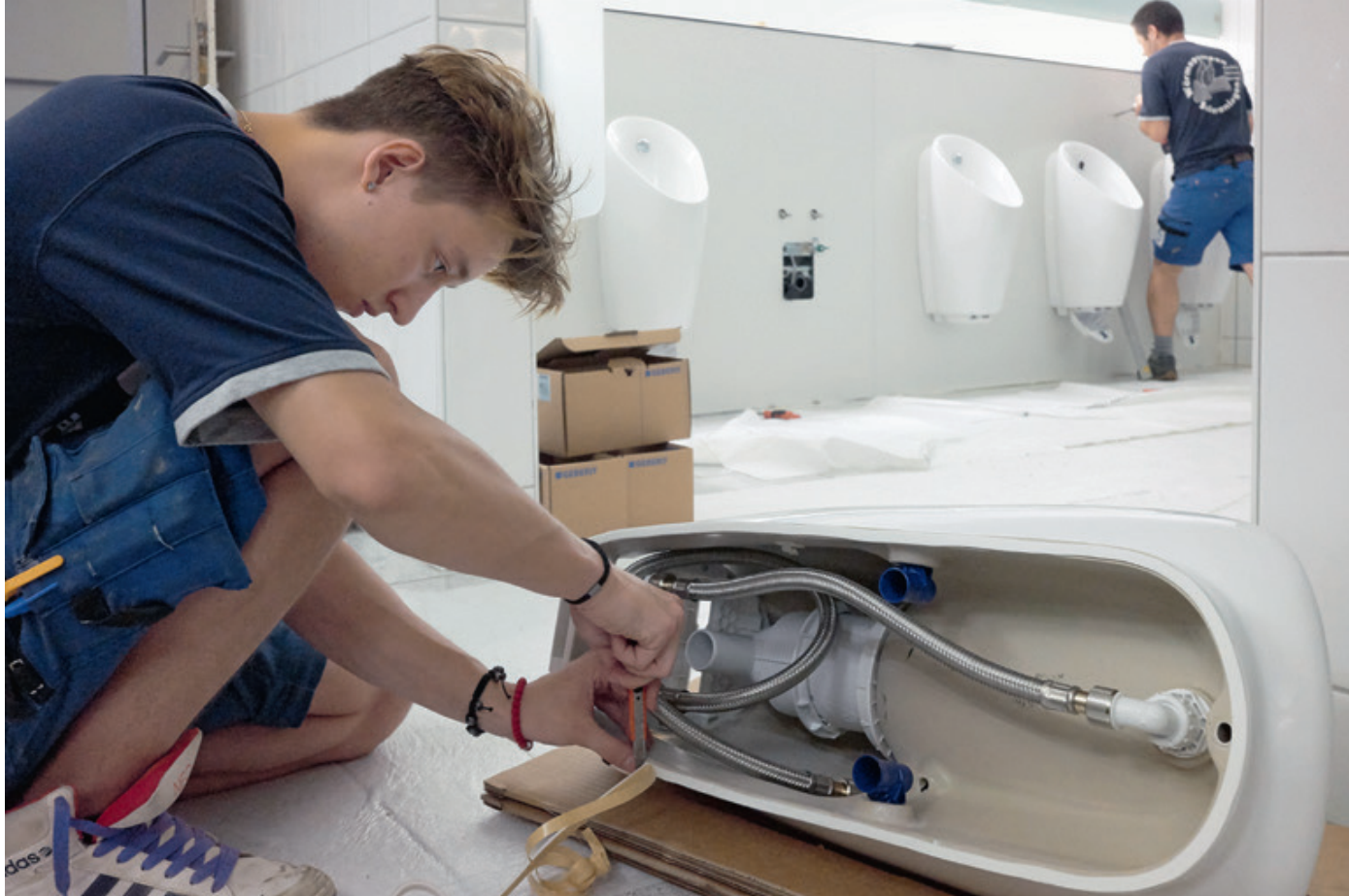
← Yannick Ramseier, an apprentice at Bürge Haustechnik AG, prepares a Geberit Preda urinal for installation. Head fitter Paul Arnold can be seen in the background installing urinal divisions.
